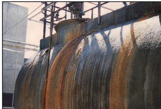
Corroded tanks, containing 98% H 2 SO 4
