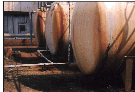
After 13+ years, only chalking and staining is evident
